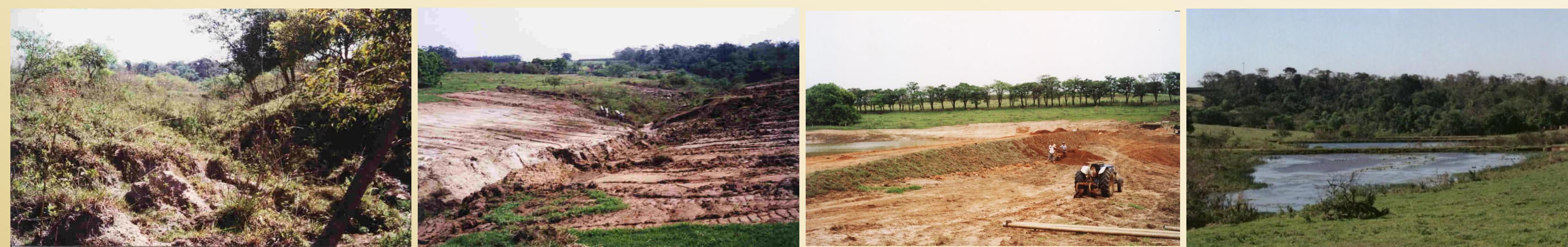
Figure 1. Gully erosion stabilization before plantation (1998)
